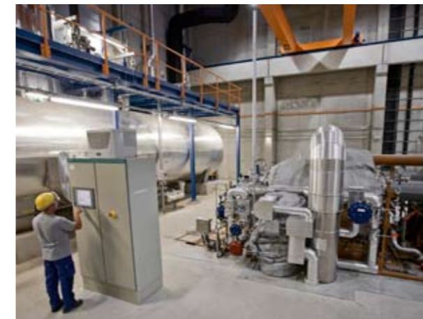
KONTROLLSTATION CONTROL STATION
